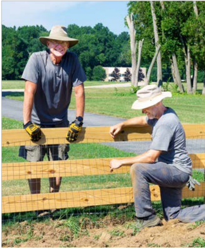
BEFORE: Rich Allen, Land Steward (l), and Dave Seiler, Land and Property Steward, constructing the Historic Garden fence.
