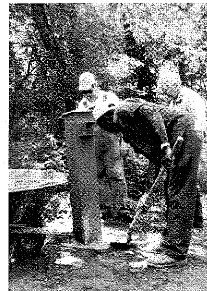
PSE&G employees, Charlie Rosani and Doug Howlett, and Jesse J. Brown of Suburban Fence install a gate at Roebling Park
