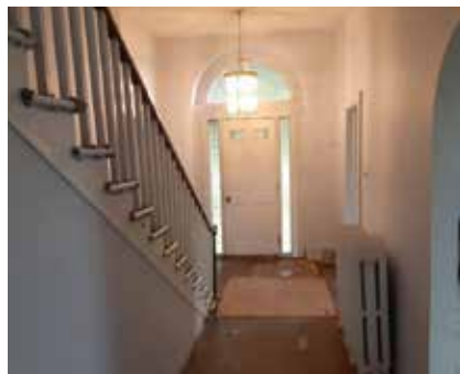
The entrance hallway shows the front door with sidelights that was in place, and the damage done to the floor from a lead under the door.
